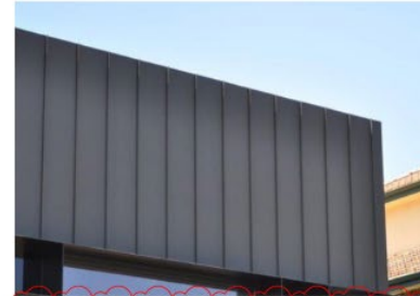
CLADDING (CL1) STANDING SEAM STEEL CLADDING WITH POWDER COAT FINISH (INTERPON D2525 SABLE BRILLIANCE MATT) - TO MATCH LVR
